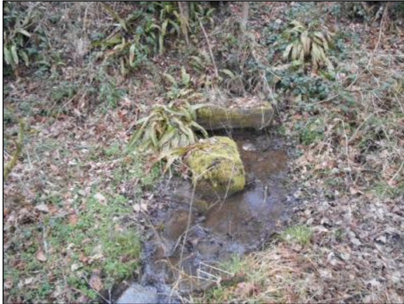
Water from road to toe area.
